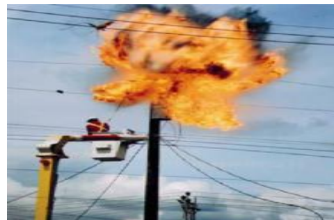
Figure 1 Faulted pole top Transformer
