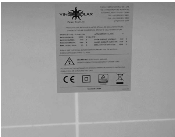
Figure 4 Solar Power Nameplate
