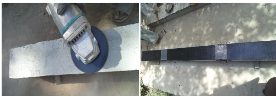
Figure 3. The surface of the beam roughened afore put on CFRP and applied CRFP Sheet on beam
