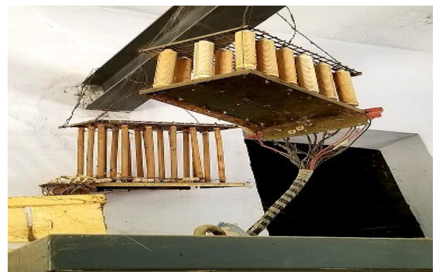
Figure. 9 Tableeghi Markaz Mardan dummy resistive load
