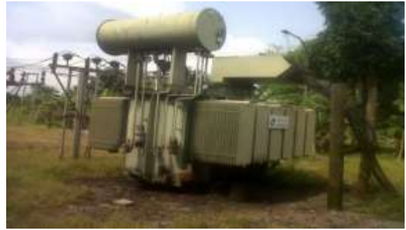
Figure1: Photo View of U-15, 15MVA, 33/11kV Injection Substation.
