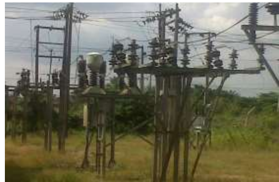
Figure 2: Photo View of U-15, 15MVA, 33/11kV Injection Substation.
